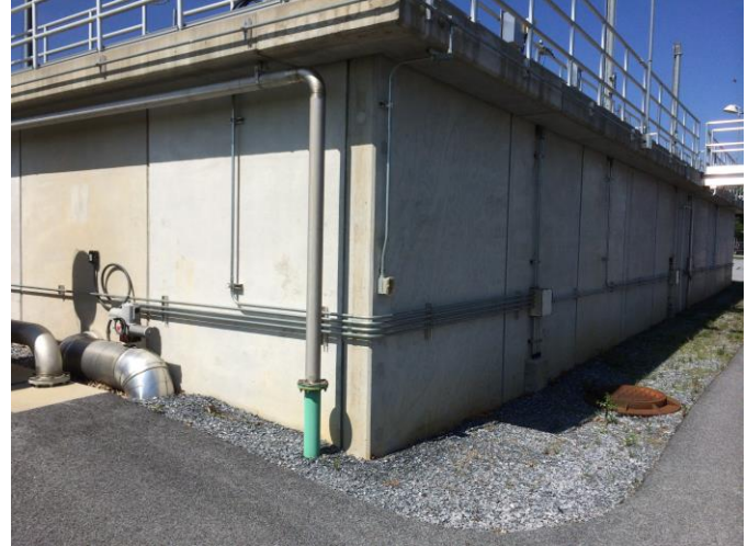
SBR Constructed in 2008 Capacity: 0.45 MGD Footprint: 109'-6" long x 41'-8" wide x 19' deep
