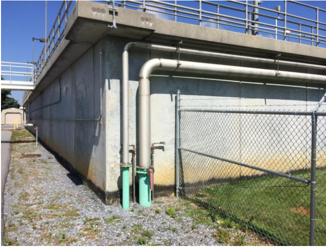
SBR Constructed in 1991 Capacity: 0.52 MGD Footprint: 127'-4" long x 41'-8" wide x 19' deep
