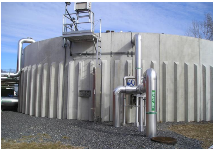
2.3 MG (BVF) anaerobic digester installed by Dutchland for Ken's Foods in 2000
